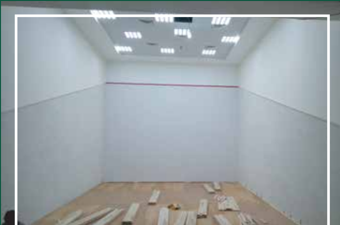
Portsaid Sporting Center Lighting Project
