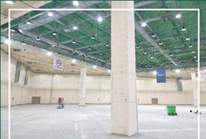
Cairo Exhibition Center Lighting Project
